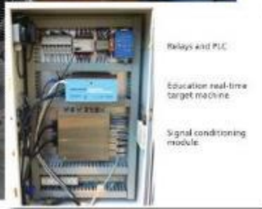
Cabinet with control system
